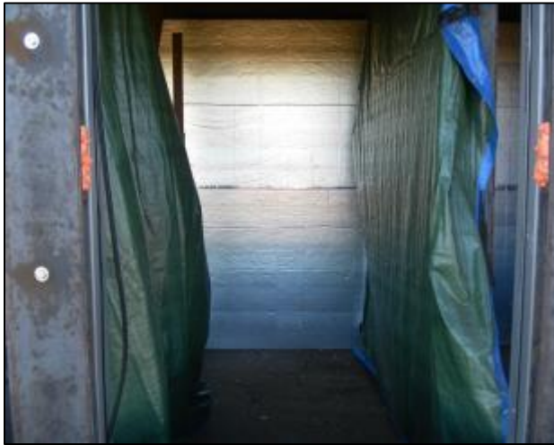
Photo No 75 Post-test, Exterior Specimen 10
