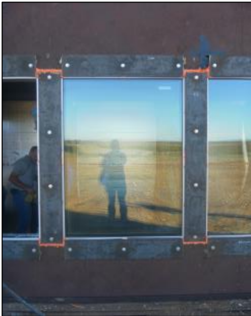
Photo No 140 Post-test, Exterior Specimen 18
