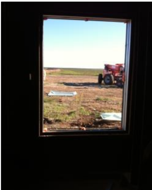
Photo No 68 Post-test, Exterior Specimen 8
