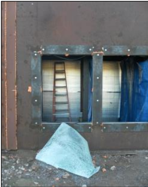
Photo No 101 Post-test, Exterior Specimen 13
