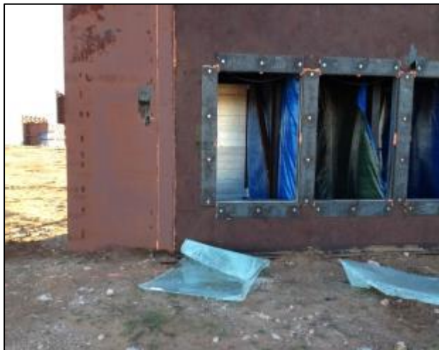
Photo No 3 Post-test, Exterior Specimen 1
