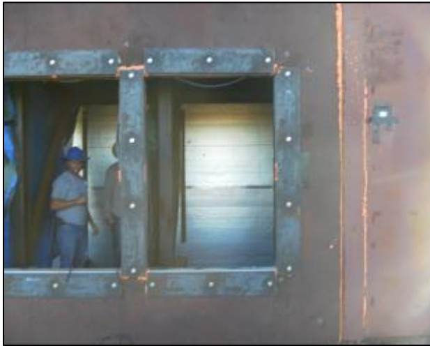
Photo No 96 Post-test, Exterior Specimen 12
